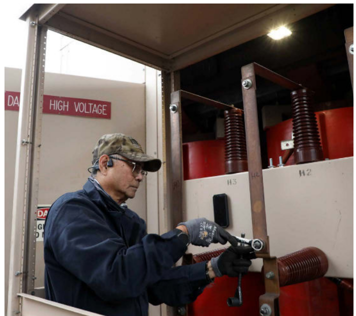
BART’s traction power substations help distribute electricity to the trains.
