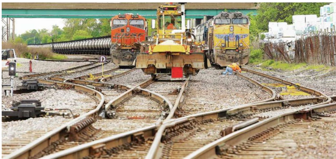
An average of 66 trains pass through the Lenox Tower interlock, which is located at the intersection of four railroads: Union Pacific, Canadian Pacific Kansas City, Norfolk Southern, and Alton & Southern. Movements were restricted by diverging turnouts and a specialty track switch known as a single slip switch.
