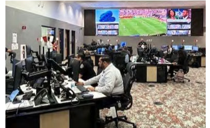
Figure 21. Emergency Security Operations Center (ESOC) Credit: LA Metro
