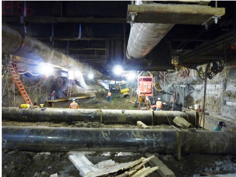
Figure 7 - 96th Street Station excavation and support of utilities under the street decking, 2nd Avenue Subway, NY
