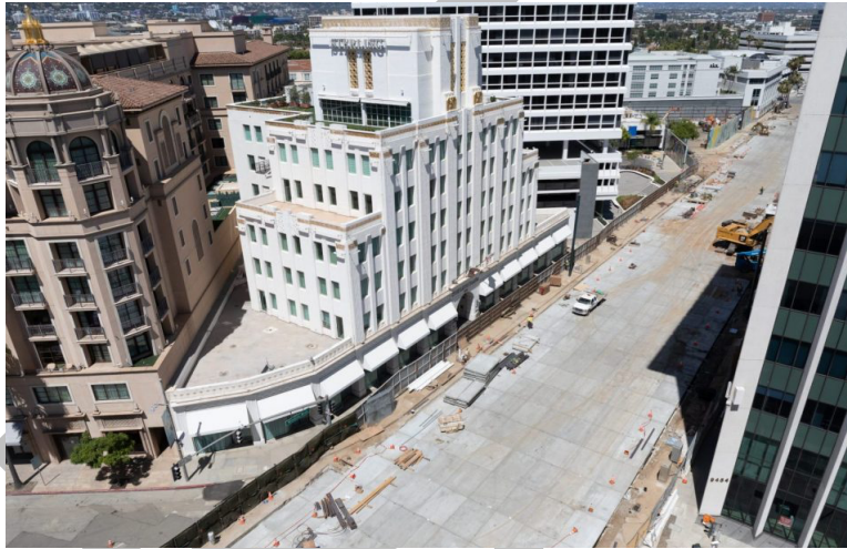
Figure 2 - Traffic Decking for the construction of Beverly Hill Station, LA Metro Purple line
