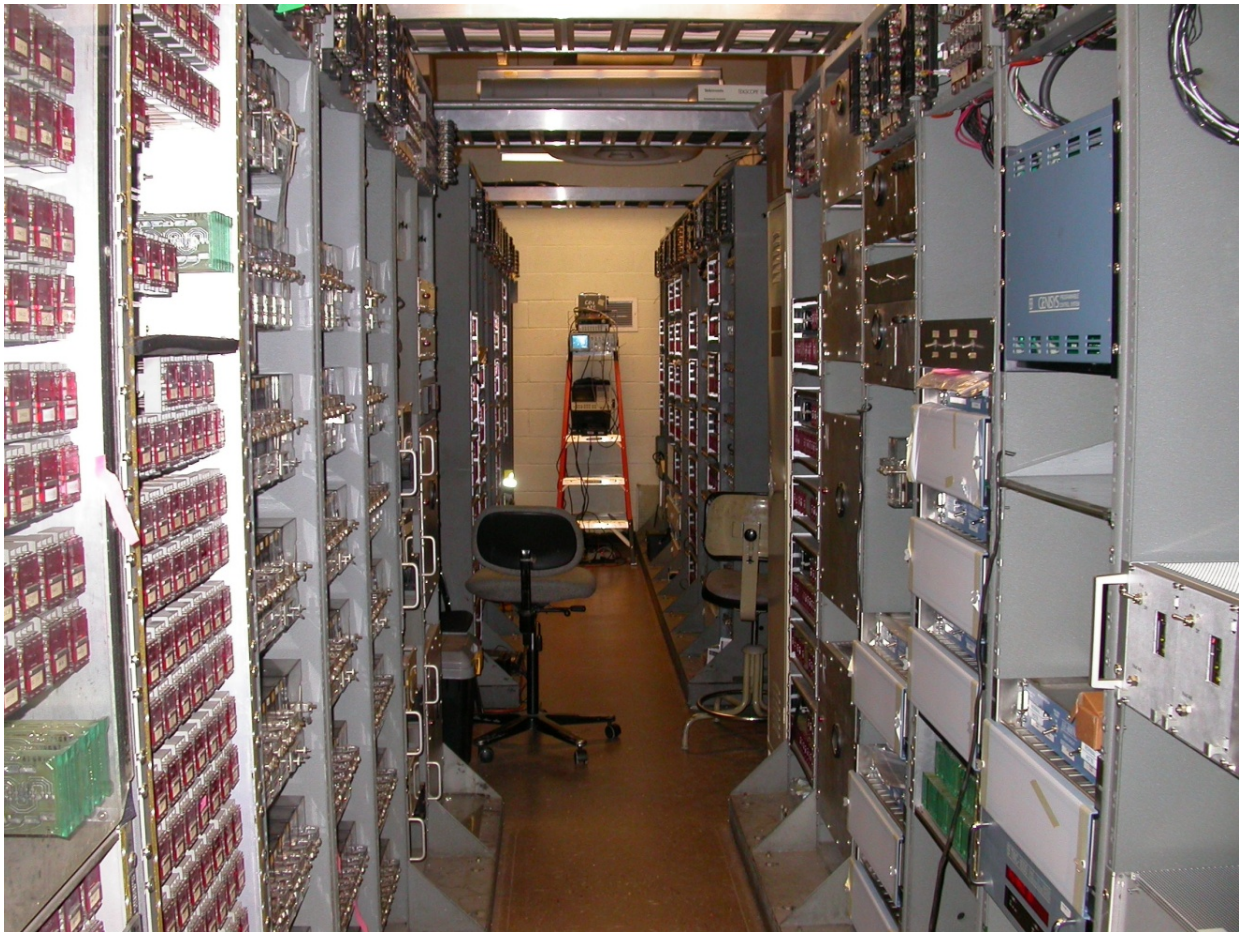
Figure 5. Racks of automatic train control components at Fort Totten train control room.
