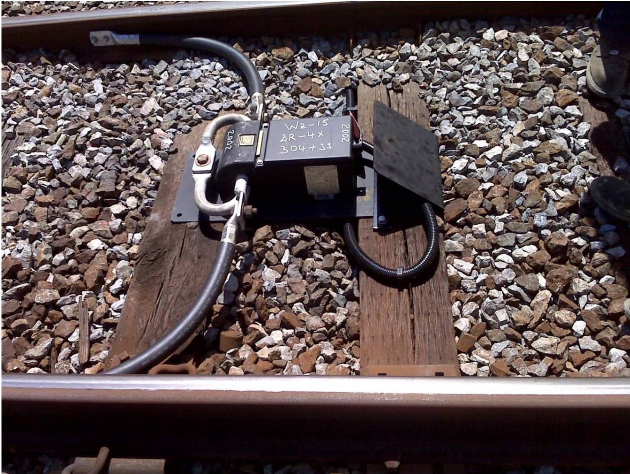
Figure 8. Impedance bond for track circuit B2-304.
