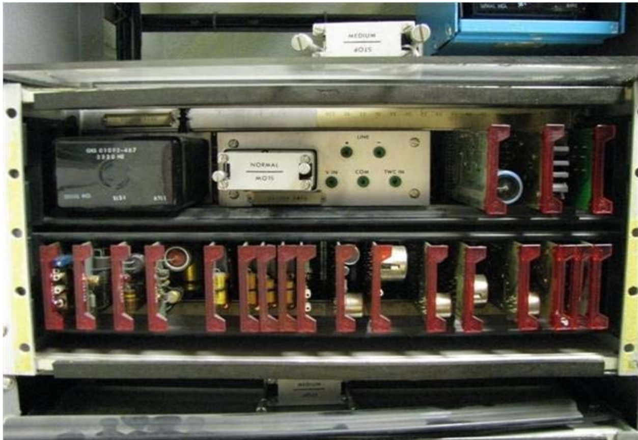
Figure 9. Typical track circuit module.
