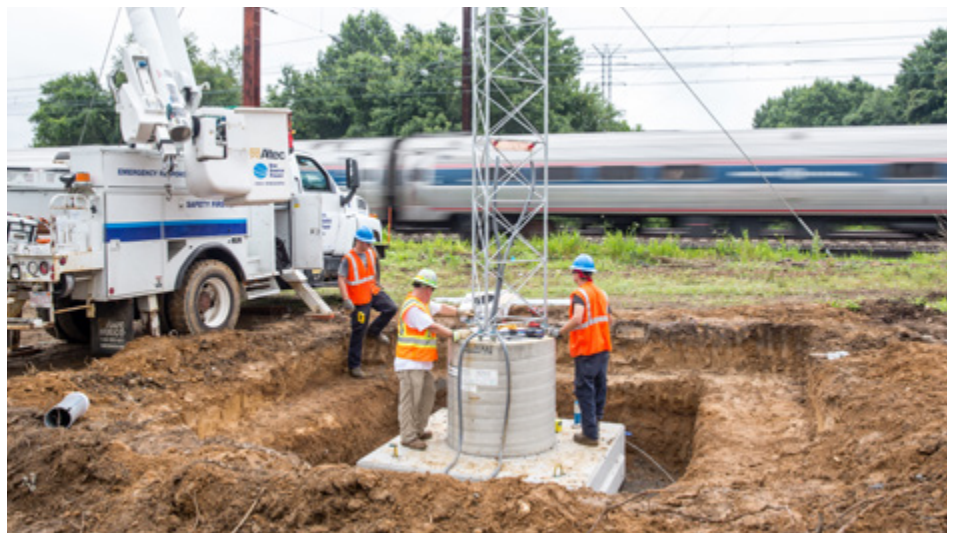
Above: Engineers installing secure trackside wireless broadband network (TSN) on Amtrak's Northeast Corridor (NEC). The purpose of TSN is to provide passengers aboard Amtrak's Wi-Fi equipped trains on the NEC with a reliable, consistent broadband-speed Internet connection.
