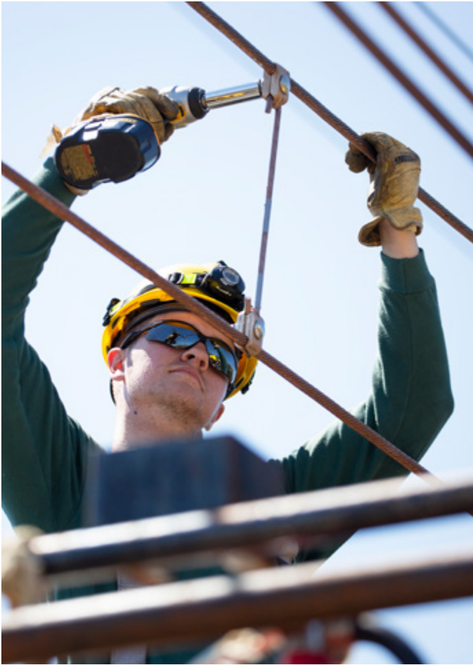
Above: A lineman of the Electric Traction team works from a Catenary Car in New Jersey.
