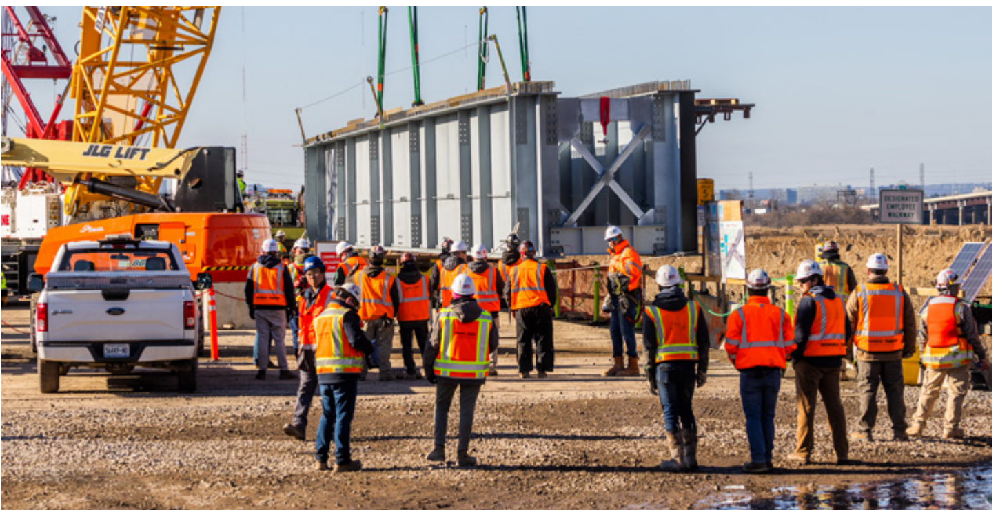
Above: First steel beam is placed on the New Portal North Bridge. Photo by Amtrak/Marc Glucksman.
