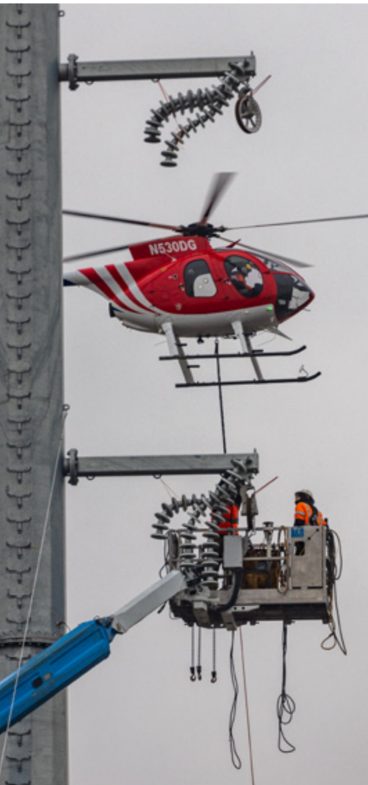
Above: A helicopter strings rope during a power transmission pole wire installation in Newark, NJ. Photo by Amtrak/Marc Glucksman/River Rail Photo.
