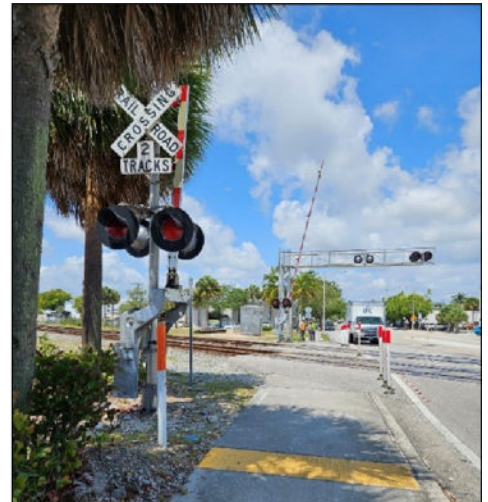
Grade crossing with a pedestrian gate. A gate arm adjacent to a grade crossing was installed to improve pedestrian safety (Fort Lauderdale, Florida).
