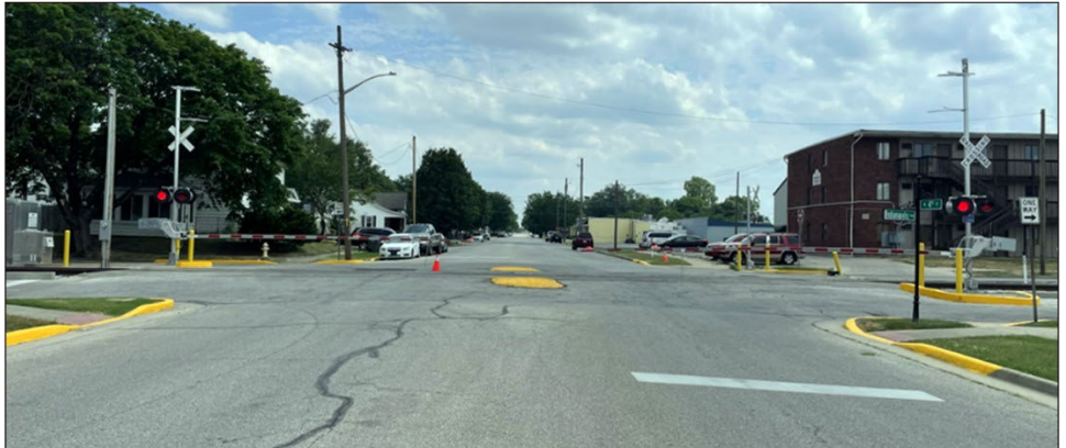
Figure 12: Completed Railway-Highway Crossings Program Project in Seymour, Indiana, That Added Gates and Flashing Lights on the Sides of the Roadway and Medians
