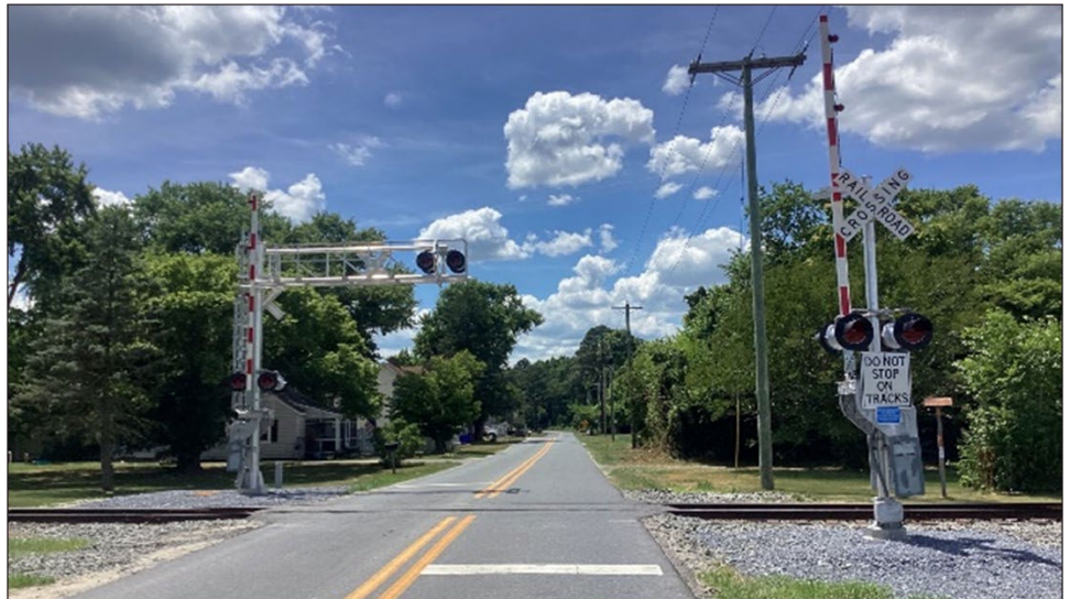
Figure 10: Completed Railway-Highway Crossings Program Project on Bacon's Road in Laurel, Delaware, That Upgraded Signals, Gates, and Lights at a Grade Crossing (#516390T)
