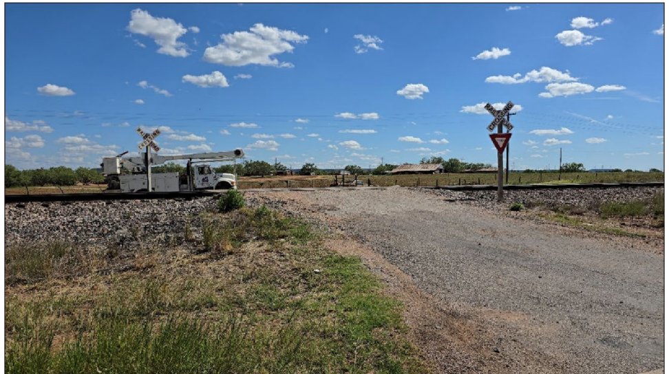
Figure 8: A Humped Grade Crossing in Trent, Texas, Prioritized for Railway-Highway Crossings Program Funded Safety Improvements
