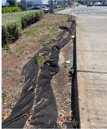
Uneven surface levels sidewalk (Hō'ae'ae, West Loch)
