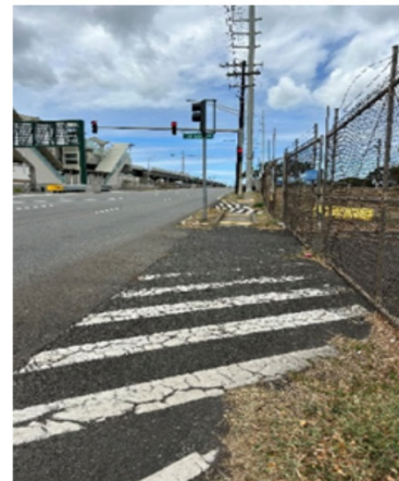
Uneven cracked sidewalk (Kalauao Station)
