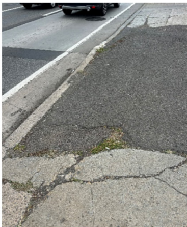
Pothole and loose gravel on sidewalk outside station (Kalauao Station)
