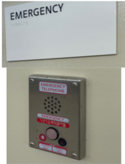
Emergency pillar at rail platform with braille
