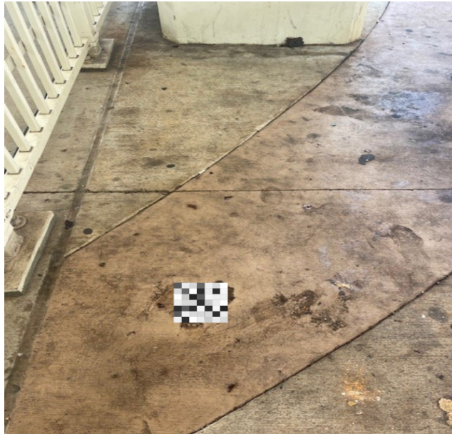
Human Feces on sidewalk under station (Hō'ae'ae, West Loch) Source: Office of the City Auditor
