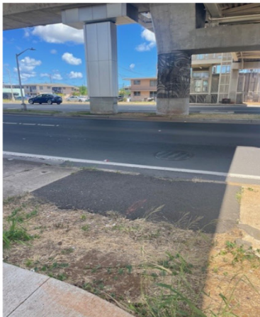
Uneven surface level on sidewalk (Pouhala, Waipahu Transit Center)
