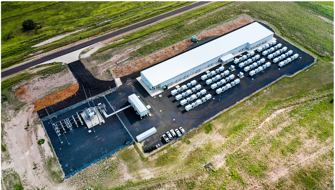
Example of Battery Energy Storage System Unit
