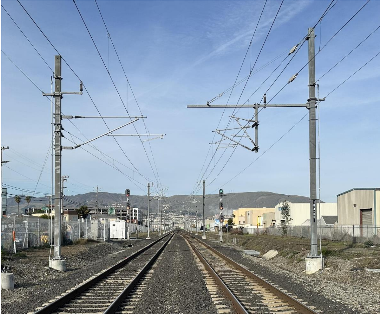
Figure 5: Photograph of Typical Double Track OCS Showing Support Poles
