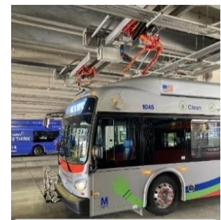
Battery-electric bus charging at Shepherd Parkway Bus Division
