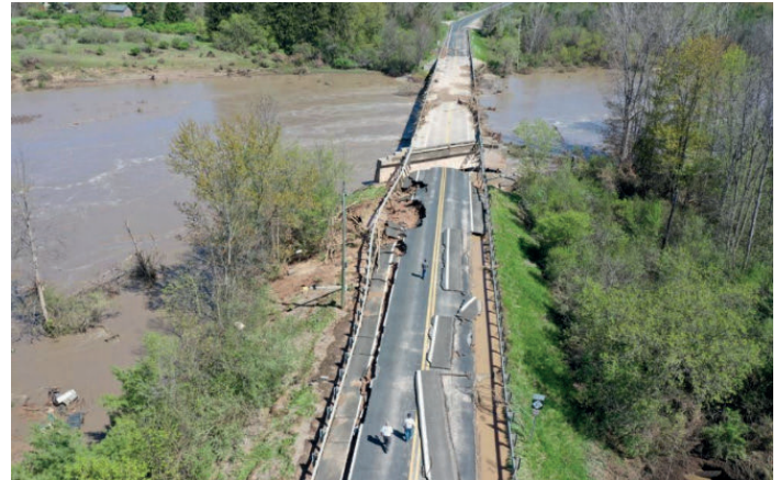
Roadway flooding and damage in Midland County
