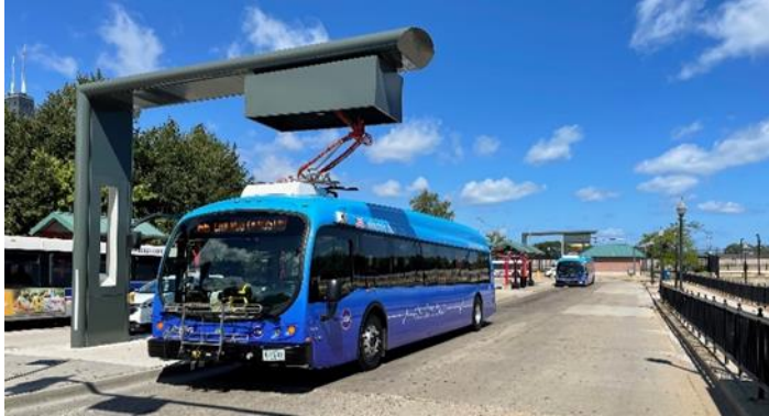
A CTA electric bus charges using the high-powered, overhead charger at the Navy Pier bus-turnaround.
