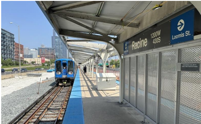
A 7000-Series train approaching the Racine Blue Line station, where work is currently underway to construct a brand new, modern, and fully accessible main stationhouse.
