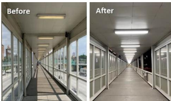
Lighting upgrade in the pedway at the Sox-35 th Red Line Station
